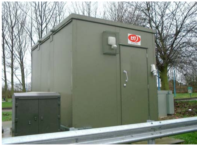
Quality REBs for housing switchgear and telecom equipment
